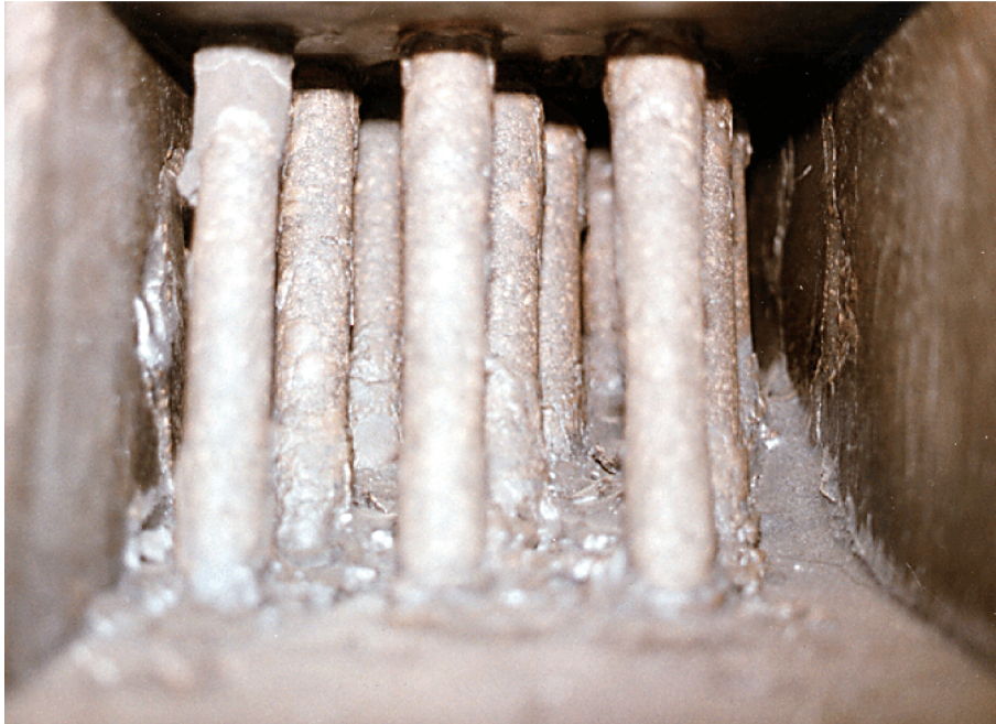
Figure 3-10. Photograph of slag screen tubes following the January test.
