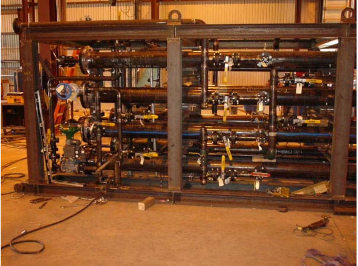
Figure 2. Photograph of the membrane skid for NTE pilot test.
