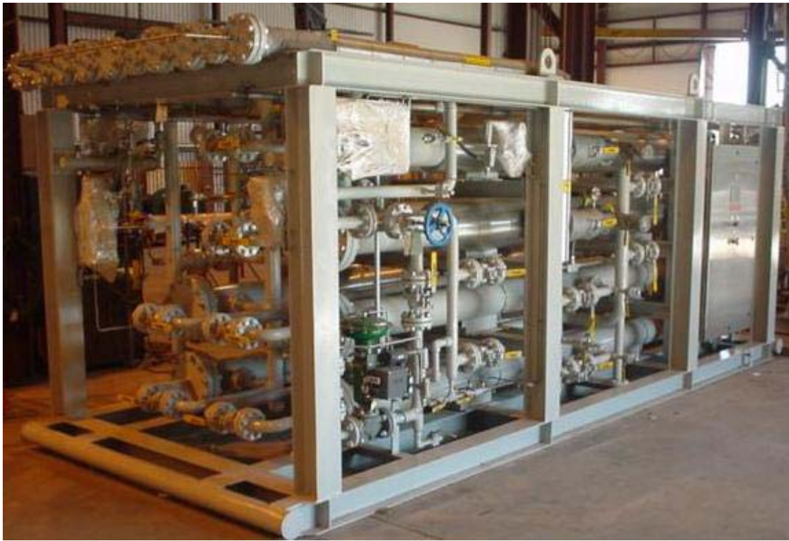
Figure 2. Photograph of the membrane skid for the NTE pilot test.
