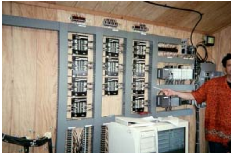
Image 7-1: Completed hardware installation
