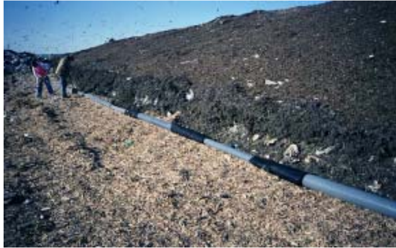
Image 3-2: Horizontal LFG collection line
