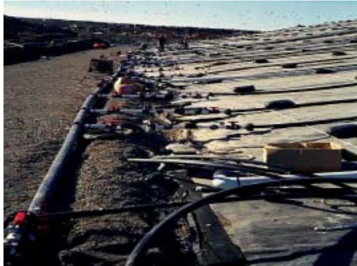
Image 3-6: Leachate injection header and laterals
