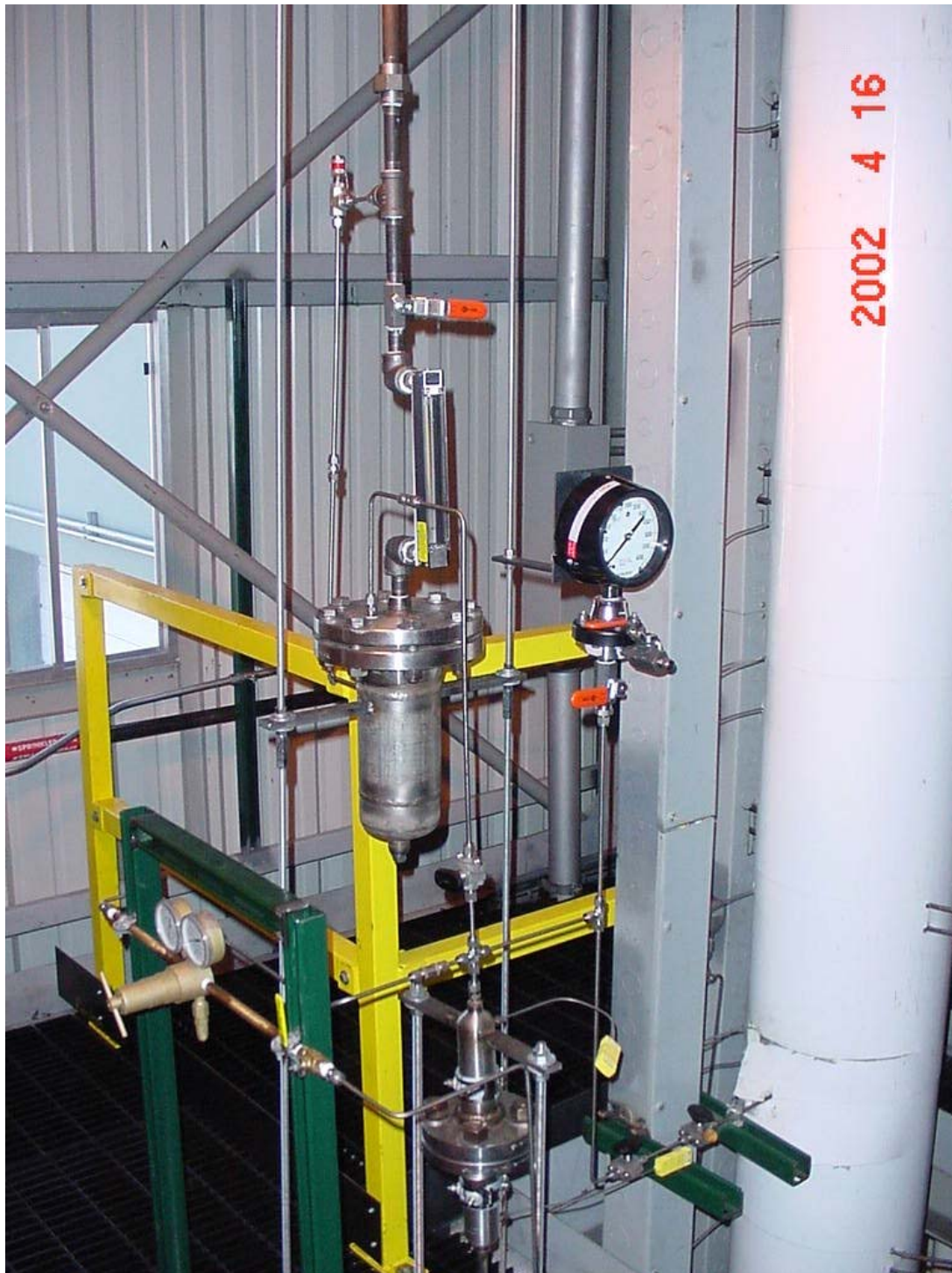
Figure VIII.C.3-4. Catalyst Withdrawal System before Insulation
