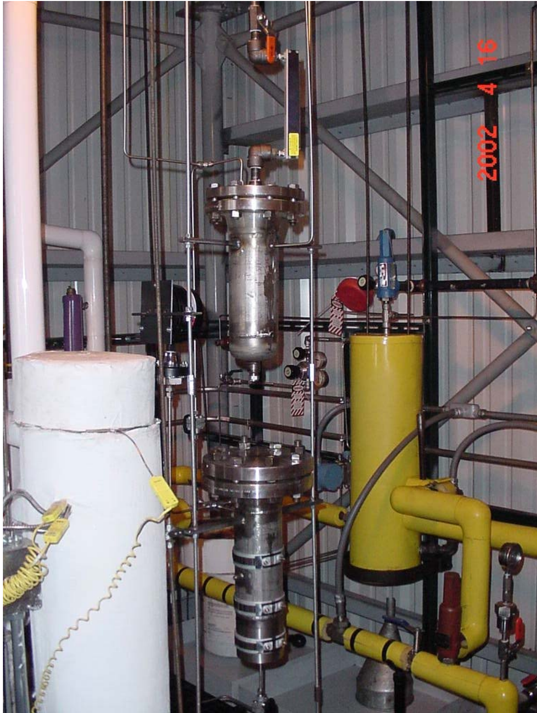
Figure VIII.C.3-3. Catalyst Addition System Hardware before Insulation
