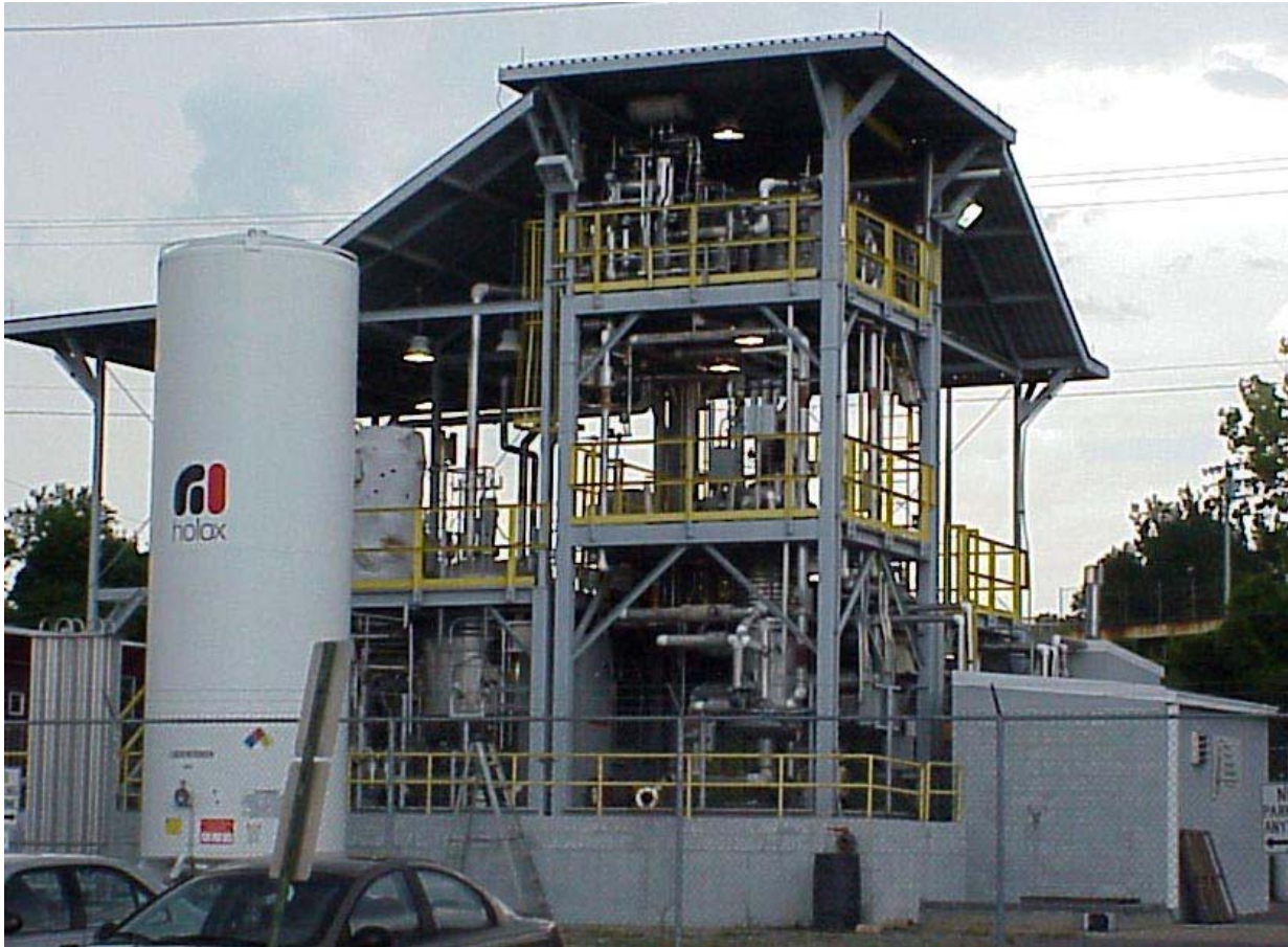
Figure 1. Filtration Research Engineering Demonstration
