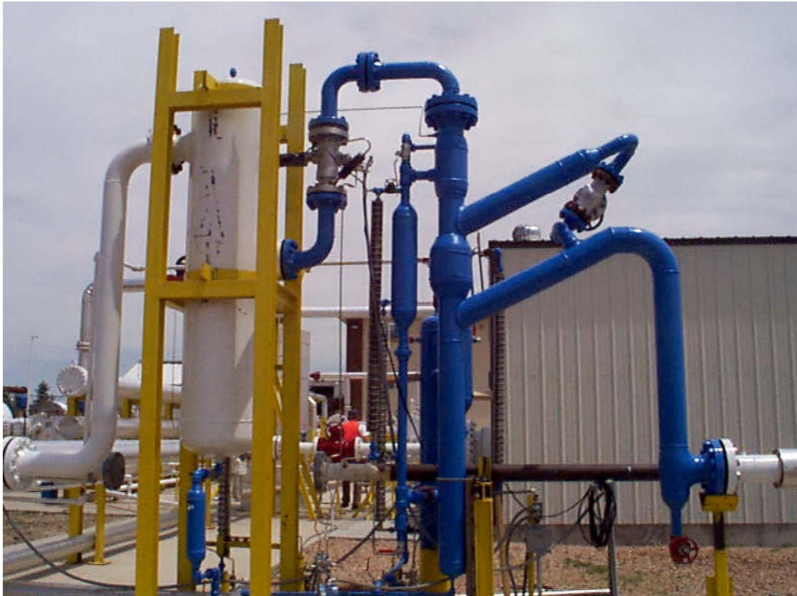
Figure 4 – High Pressure GLCC Test Facility at CEESI
