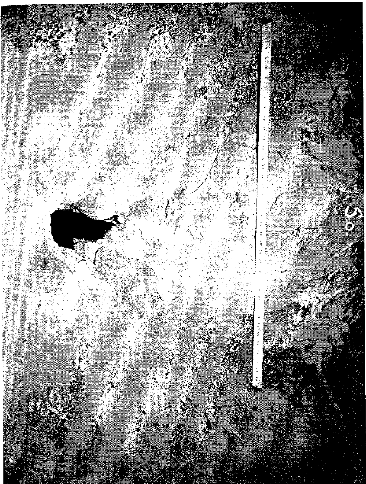
Figure 27. - South section of gasifier floor at entrance of south ash leg.
