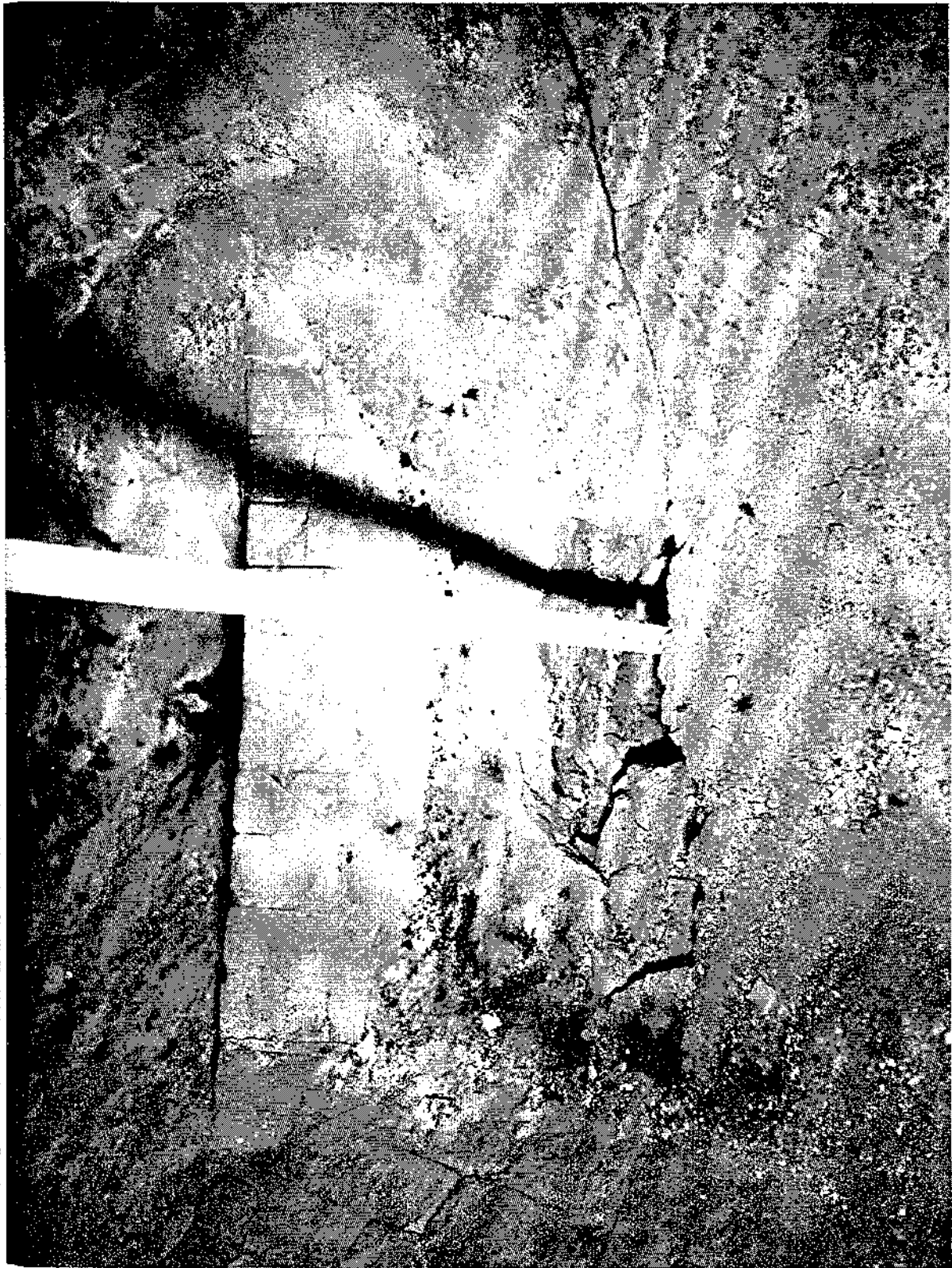
Figure 26. - Center section of gasifier floor at entrance of center ash leg.
