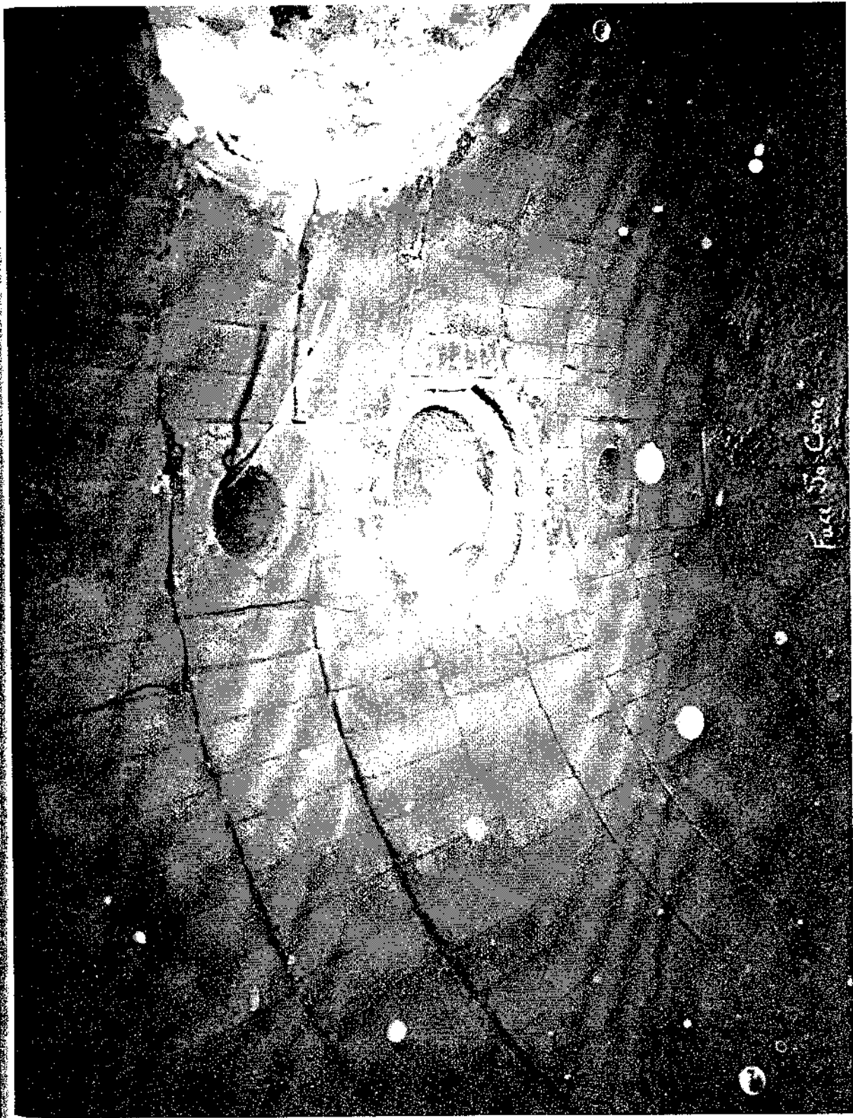
Figure 24. - Top center section of gasifier, south view.
