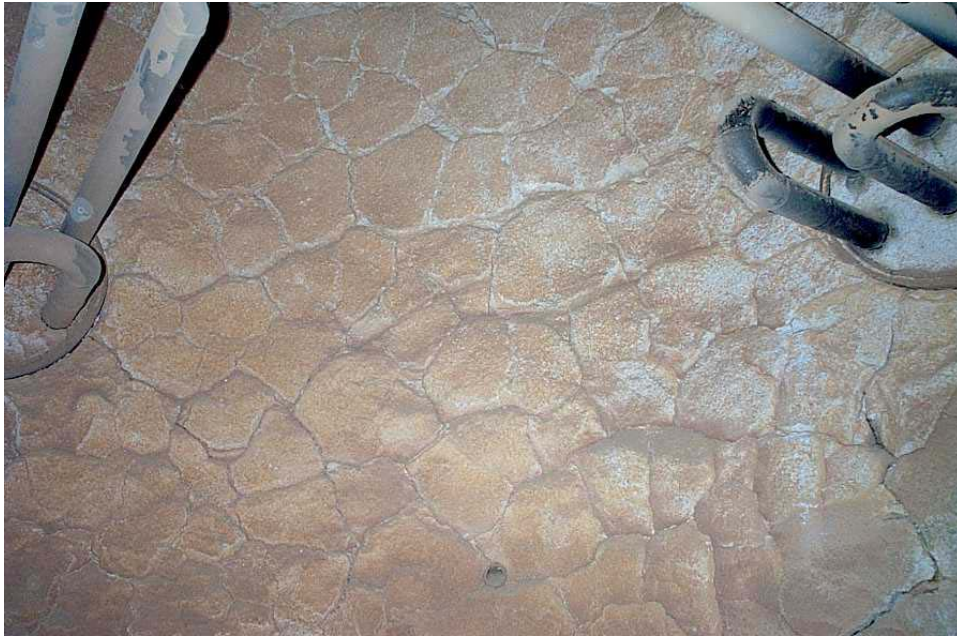
Figure 4.1-1 – View of Western Side of Sulfator Showing Cracks
