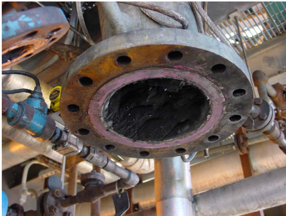
Figure 3.3-31 Drop Pipe Between FD0502 and FD0520
