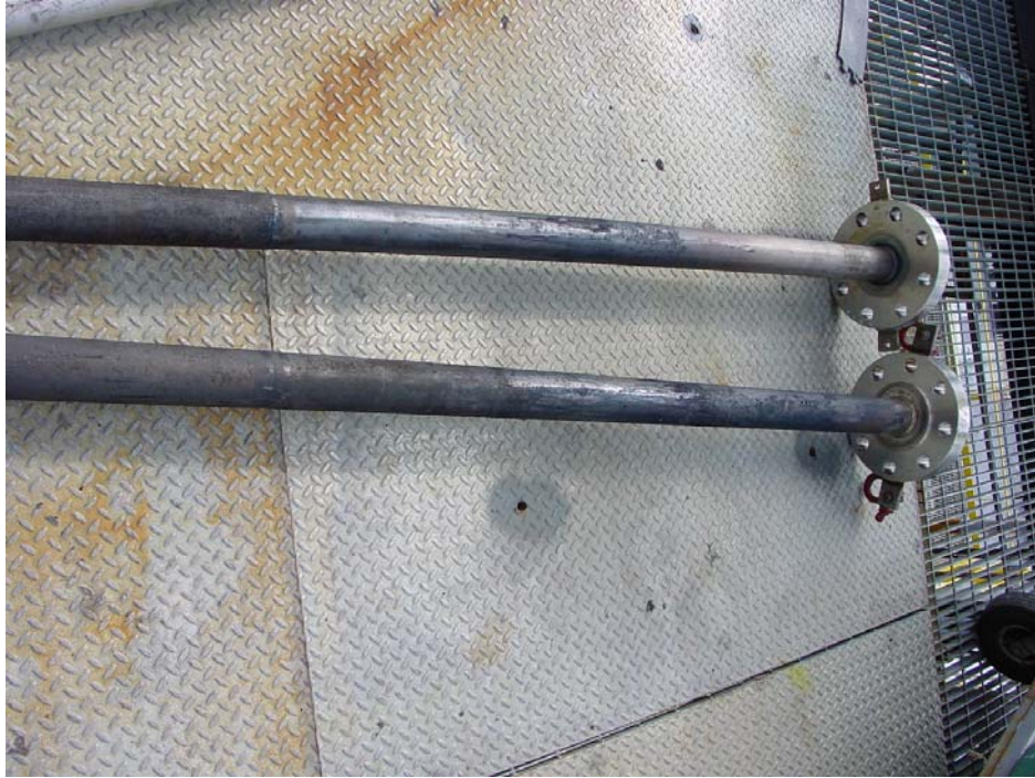
Figure 3.3-27 Back-Pulse Pipes After TC06B
