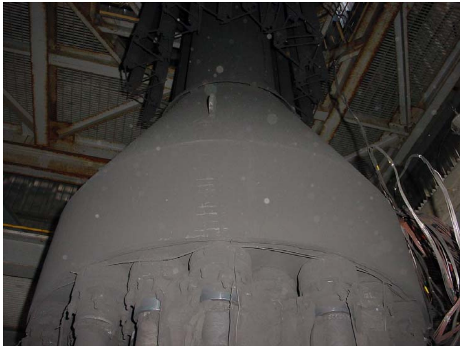
Figure 3.3-22 G-ash Buildup on Bottom Ash Shed
