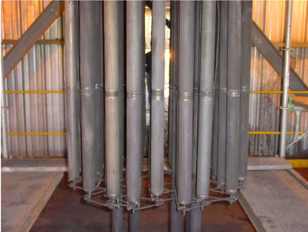
Figure 3.3-18 Filters After Being Cleaned With Air
