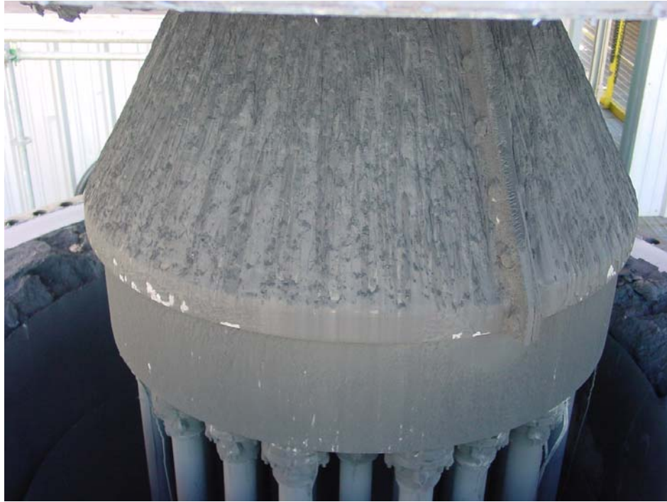
Figure 3.3-21 G-ash Buildup on Top Ash Shed
