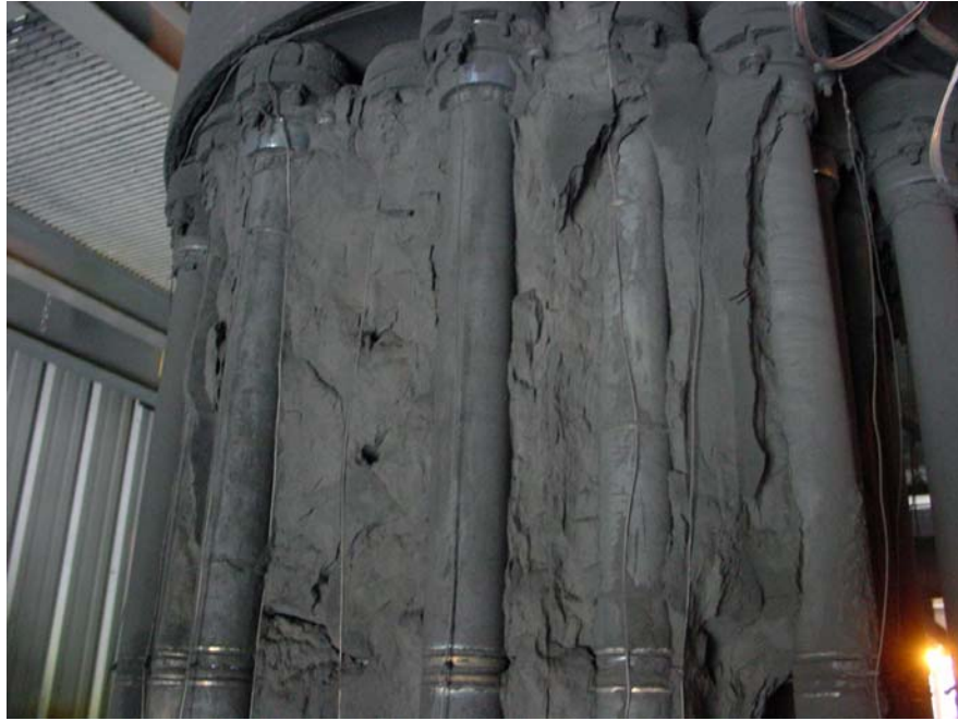
Figure 3.3-19 G-ash Buildup on Filter Element Fixtures
