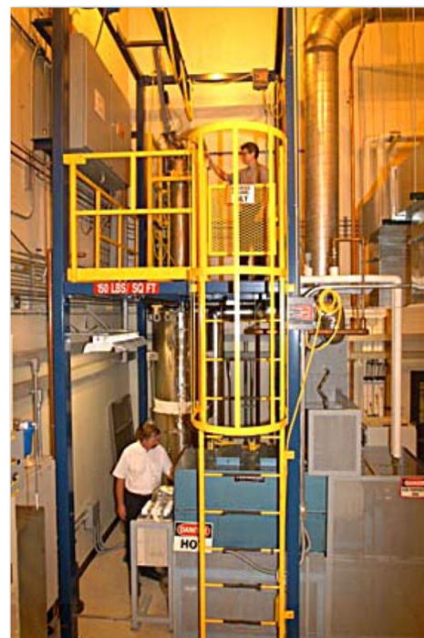
Technology Development Unit (TDU) Installed at Air Products
