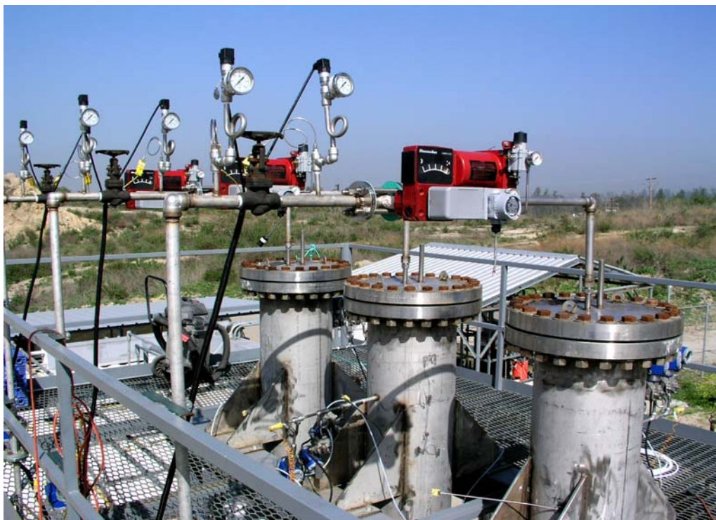
Figure 4. Photo of installed top reactor flanges as well as reactor exit piping and instrumentation.
