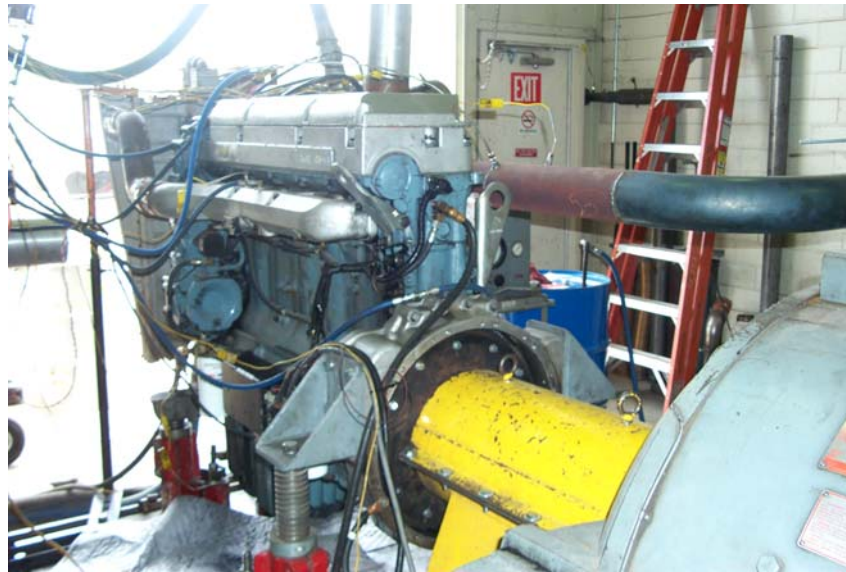
FIGURE 1. 1991 DDC SERIES 60 ENGINE INSTALLED IN TRANSIENT TEST CELL 16
