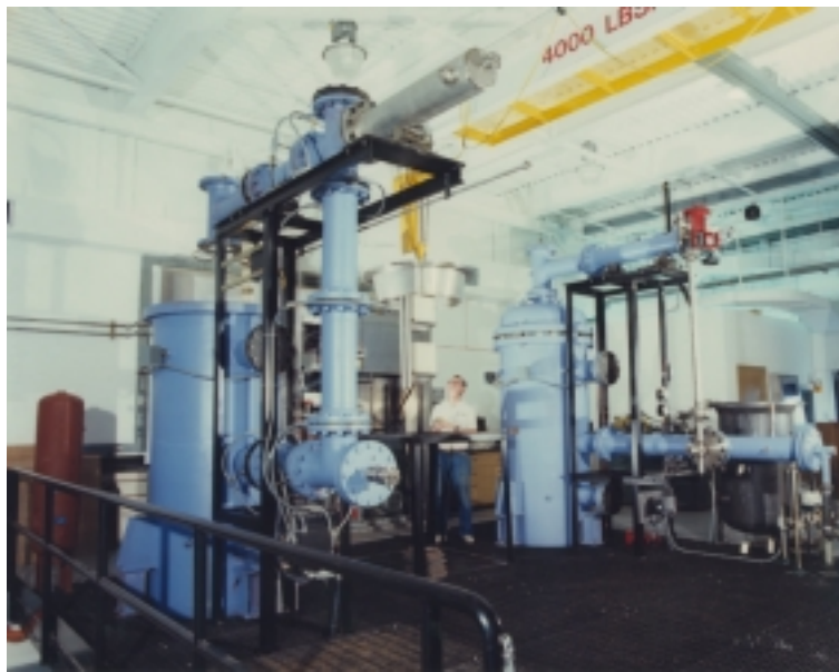
Figure 3.1 — Siemens Westinghouse PFBC simulator test facility.
