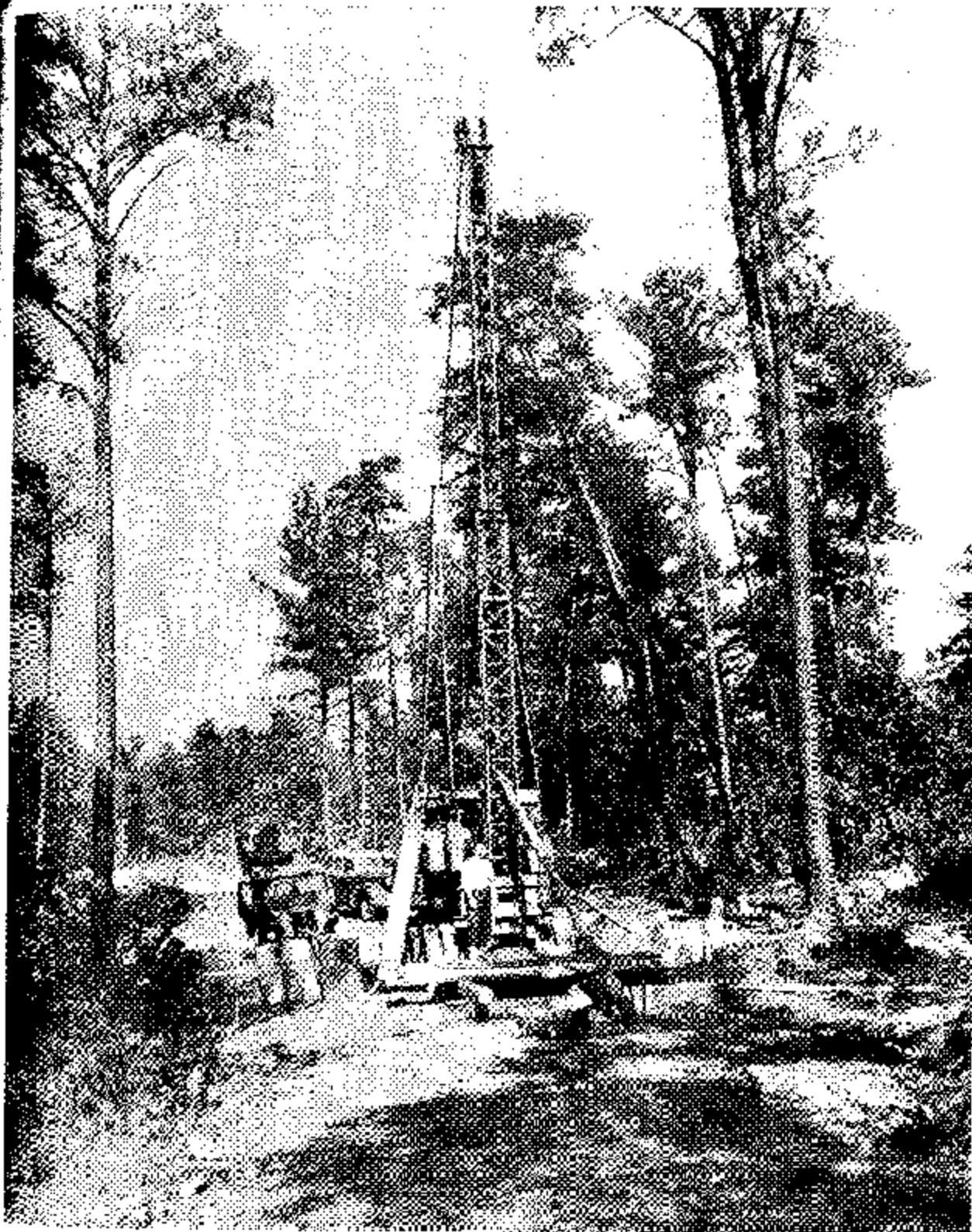
Figure 48. - Rig used to drill No. 1 churn-drill hole. Note 16-inch bit in foreground and baller standing upright at left of rig.
